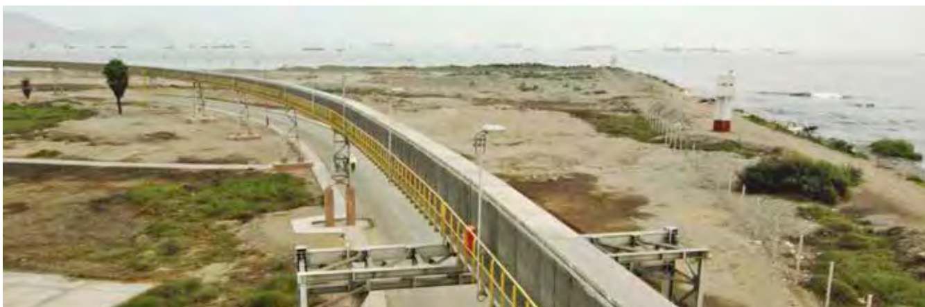
Impala Terminals' jointly owned covered conveyor belt expansion at the Port of Callao, Peru.
